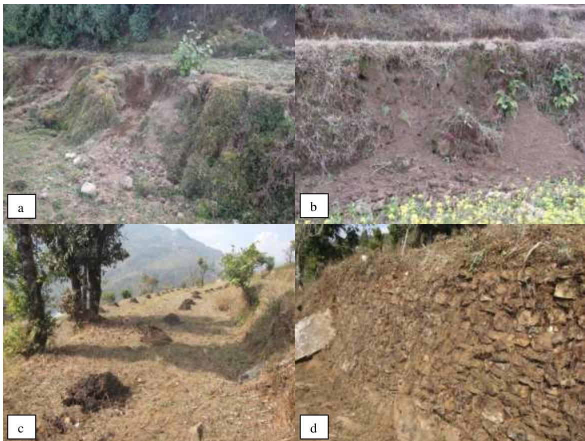
Fig. 3: Terraces are usually well maintained. Damages on terraces, whether abandoned or not, are rare. a) animal trampling on abandoned terraces, b) mice holes in terrace riser, c) application of manure, d) terrace riser reinforced with stones (Photos: G. Schwilch)
