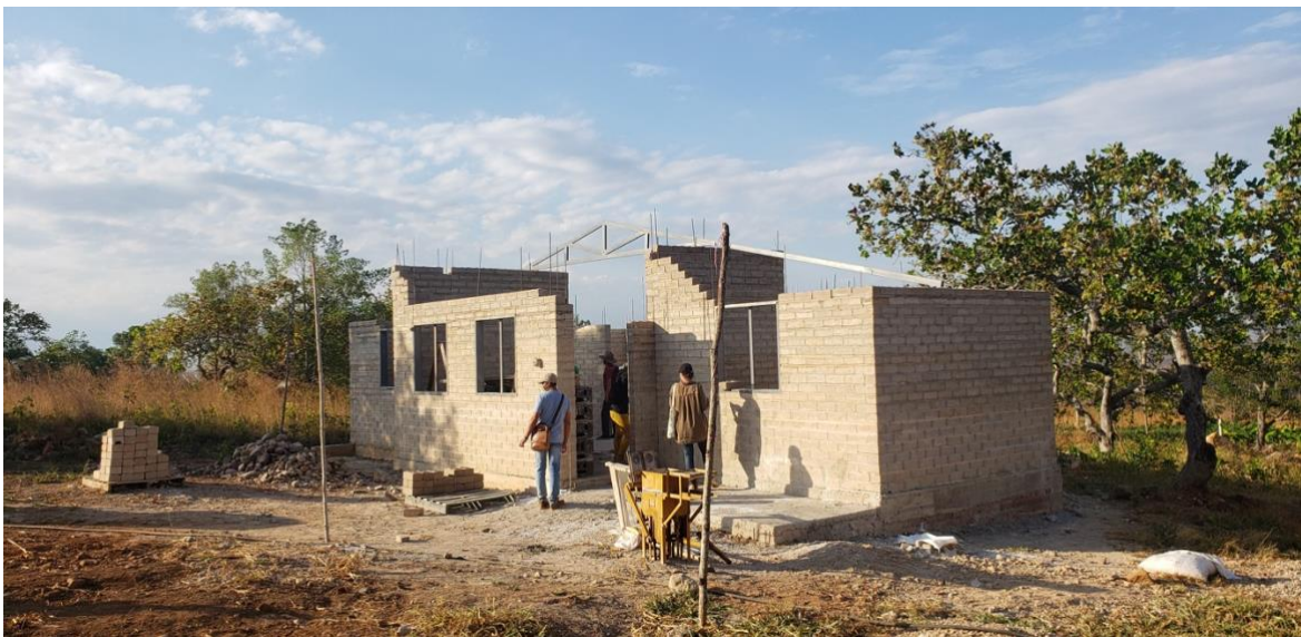
Figure 4: The community of Tierra Grata and Pandores have built two model houses where they have tested the productive units and different construction elements. Photo: Ramón Bermúdez
